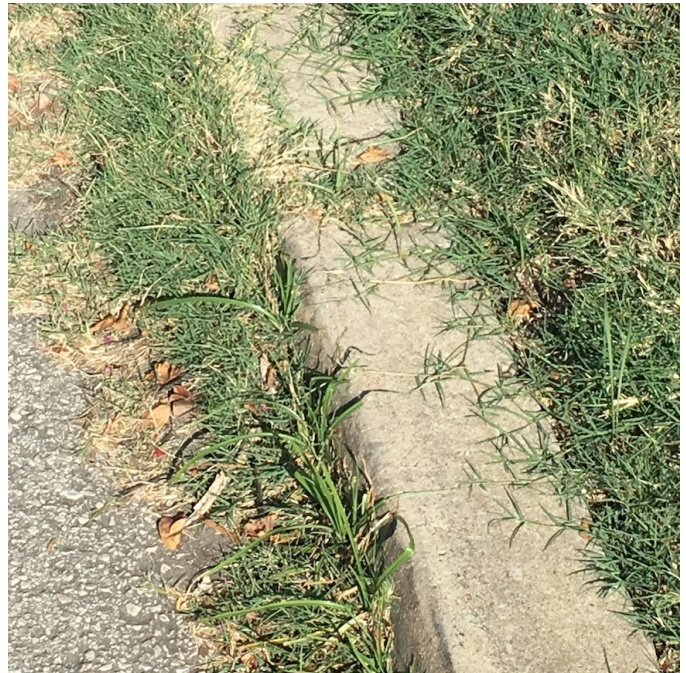
A curb lacking proper maintenance
